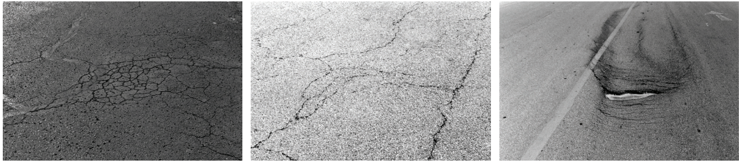
Figure 5. Different types of asphalt ‘cracking’: fatigue ‘alligator’ cracking, block cracking, and slip-page cracking
